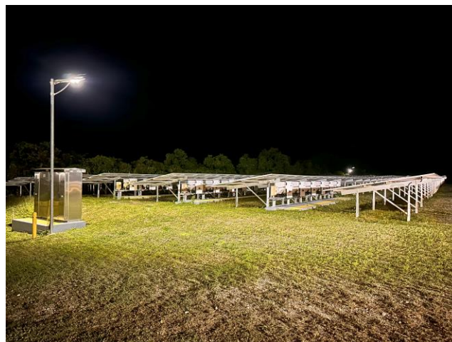
Figure 1: Munda Solar Farm
