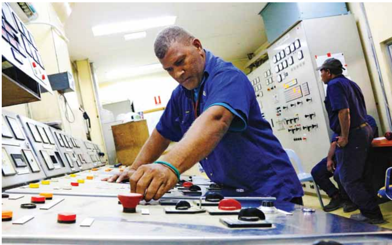
Monitoring the electricity supply at the Lungga Power Station.
